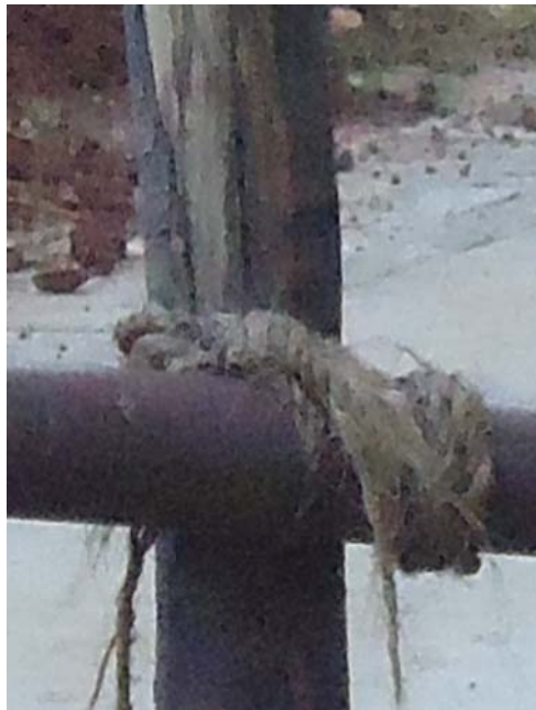
Figure 3 Scaffolding tied together as shown in Figure 2 (see online version for colours)
