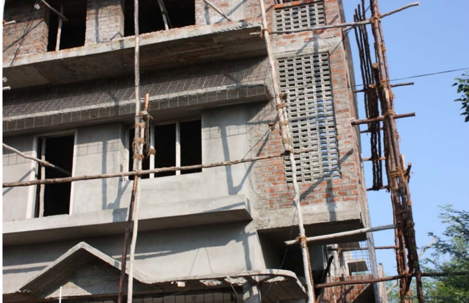
Figure 2 Scaffolding constructed of bamboo, tree limbs and rope (see online version for colours)
