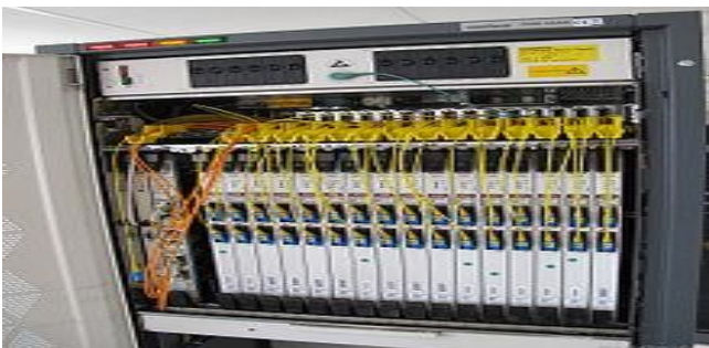
Figure 2 Optical line terminal
